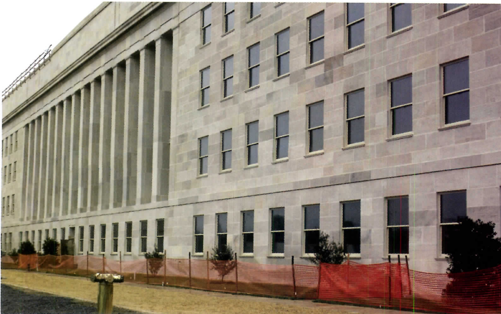
Portions of the limestone exterior of the Pentagon had to be reinstalled following the terrorist attack of September 11, 2001.
