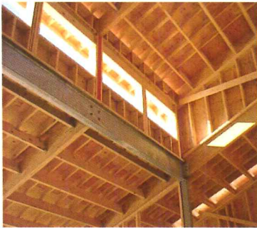
Clerestory windows help provide balanced day lighting. Environmental Experiment Center (EEC) at the Science Museum of Minnesota in St. Paul.
