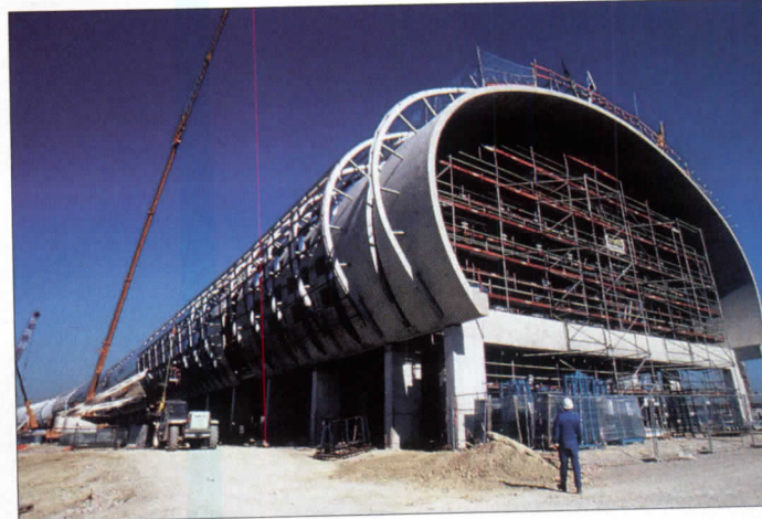
AdP had problems with the concourse's supporting columns during construction.
