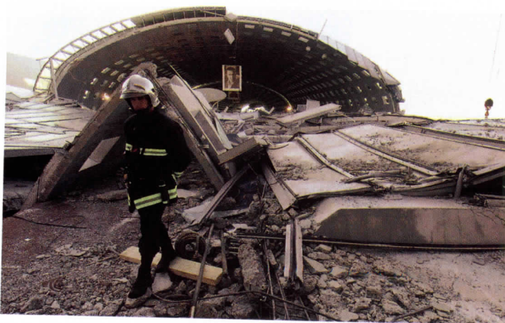
Workers are collecting debris that may point to the cause of the accident.
