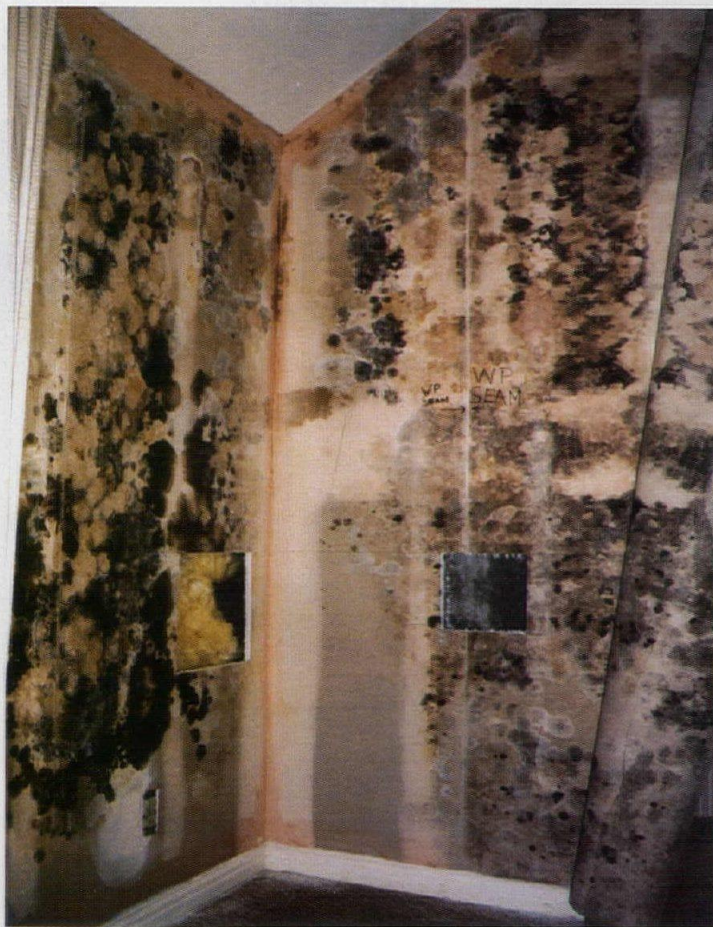
Mold flourishes on wallboard behind impermeable vinyl wall covering in a Florida hotel. Condensation forms when moist warm air from outdoors meets cooler spaces indoors. The vinyl traps the water, which is key to mold growth.
