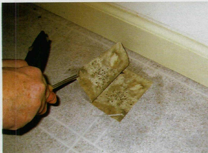
Mold grows under sheet vinyl covering a concrete floor in the Midwest because a vapor barrier had not been placed below the slab during construction, thus allowing ground moisture to penetrate the concrete.
