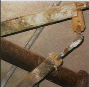
Moisture control is the key step in halting mold growth in buildings (171).
