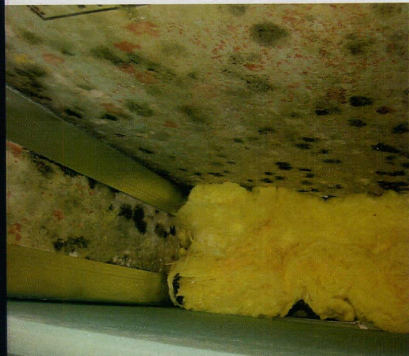
A wall cavity in a building under construction in the Northeast developed mold because materials were not kept dry prior to installation and water was entering from upper stories as they were being built.
