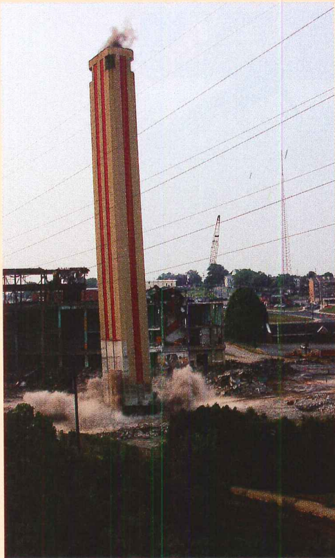
The 200-foot-tall smokestack at the Nashville Thermal Transfer Corporation facility was brought down using controlled
