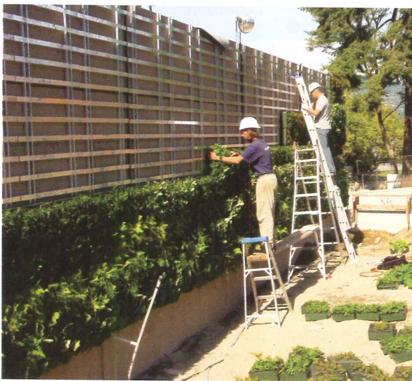
Polypropylene boxes containing pregrown plants such as flowers, mosses, and berries compose the vertical garden at the Vancouver Aquarium. A stainless-steel support grid secures the boxes to the building's structural poured-in-place concrete wall.
