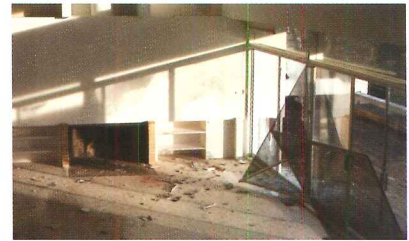
Nepal Asatthawasi (left) stands amid the rubble of Paul Rudolph's Michaels House (above). The Cerrito residence (top) is next on the list of properties facing demolition.
