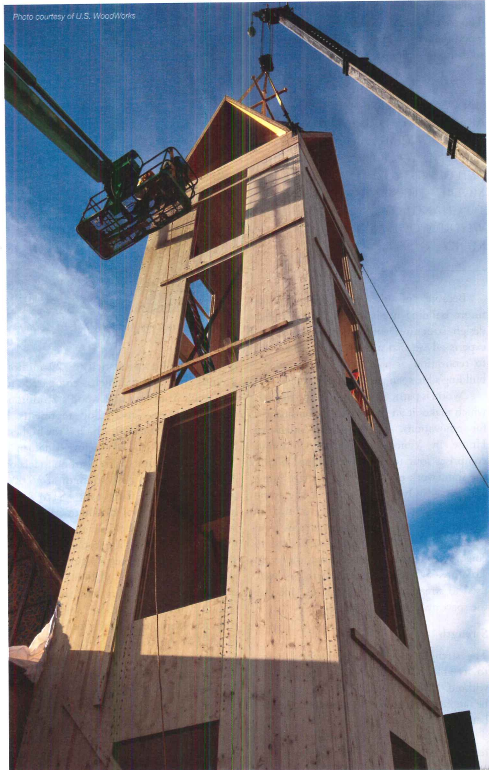
A 78-foot bell tower at Myers Memorial United Methodist Church in Gastonia, North Carolina is the first non-residential structure in the U.S. to be built from cross laminated timber.
