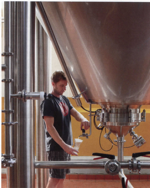
ON TAP. Workers can sample beer via spigots at the tapered base of each tank (left). Each 40-foot-tall tank has a 300-barrel capacity, and is accessed by way of a staircase on the southeast wall (right) that leads up to a steel-grate catwalk. Employees can then add anti-clouding agents and other ingredients to each vat.
