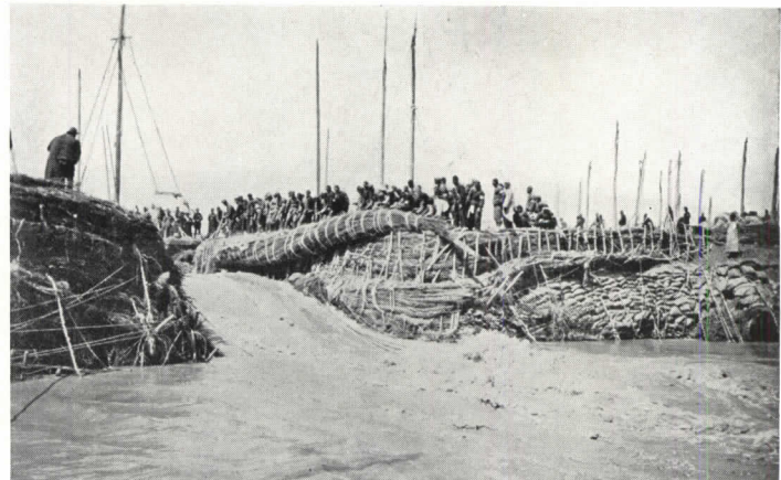
WHERE MODERN MACHINES COST MORE THAN COOLIE LABOR men push and roll the willow "sausage" to its final resting place as their ancestors did thousands of years ago. As the gap is narrowed, the rush of the water is greater, but the "sausages" are firmly fixed by rope and sticks.
