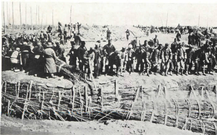
IT TAKES ONE HUNDRED MEN to roll the "sausage" to the gap. When the fascines are set in place one above the other, they are spiked and tied together with rope, and then covered over with earth and rocks.
