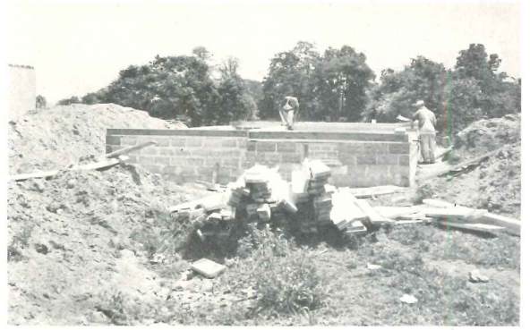
ON THE JOB: Foundations are put in, pre-cut joists set in place.
