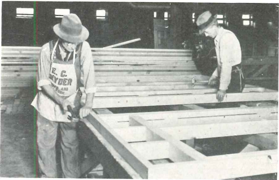
Fabrication of wall and partition units are framed from working drawings, doors and windows integral.
