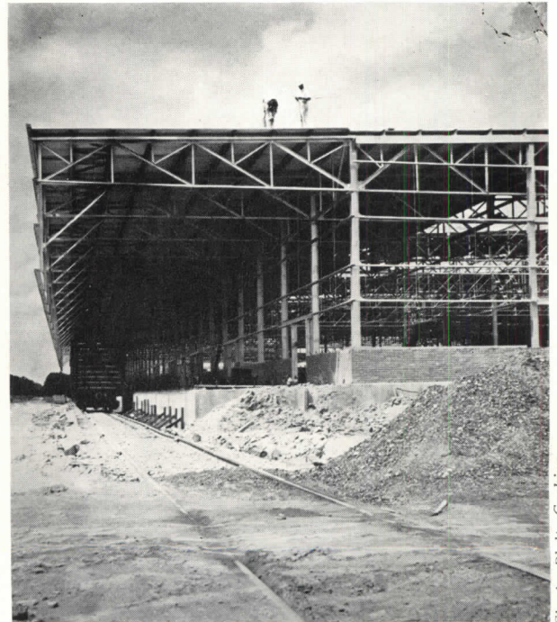
Position of suspended apron provides weather protection for men and materials. Note cantilever trusses.
