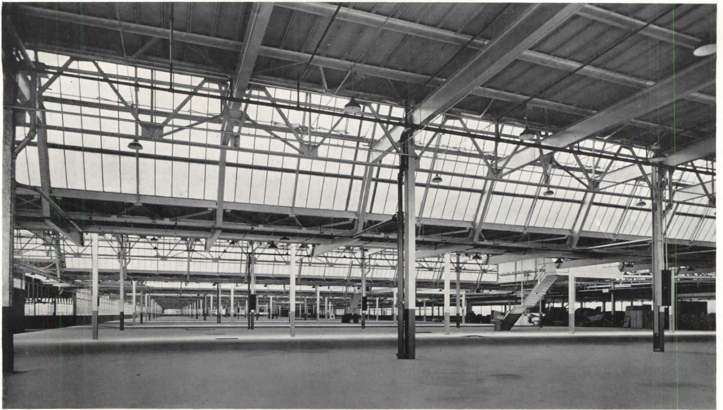
Wide column spacing—40 by 60 ft.—leaves floor space unobstructed and promotes flexibility in plant operation. By designing roof beams as cantilevers over supporting columns the weight of structural steel per sq. ft. is no more than would be required if column spacing were 40 by 30 ft. Picture shows part of the interior of the Dodge Truck factory in Detroit for which Albert Kahn, Inc., was architect and engineer.
