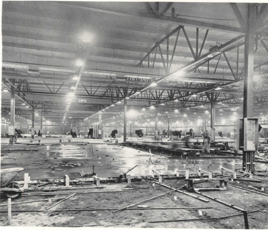
Under-floor installation of utility ducts and pipes allows greater flexibility in the economical layout of machinery and material-handling equipment.
