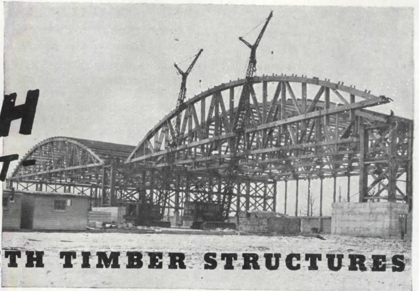
CLEVELAND. 200' laminated trusses were designed, prefabricated and erected by Timber Structures, Inc. for 200'x440' assembly plant, for The U.S. Engineers. Front trusses, (supporting doors and roof), were built to carry 450,000 lbs. Intermediate trusses built to carry 310,000 lbs.
