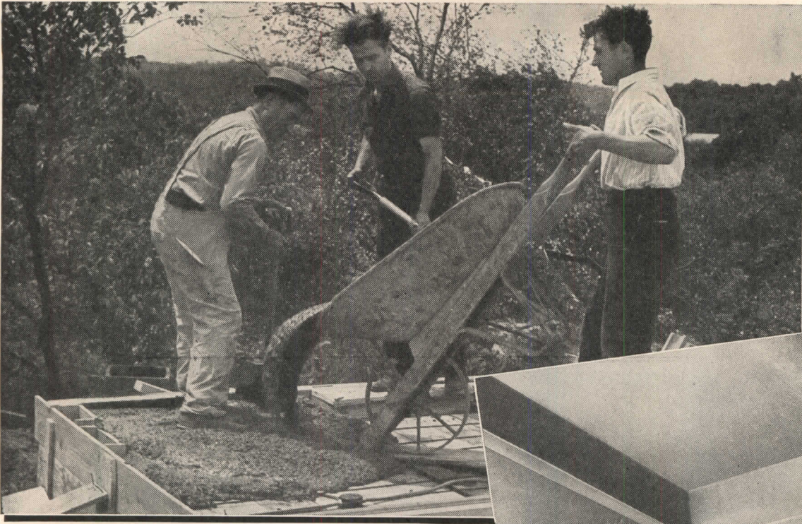
Pouring concrete to encase the ends and top flanges of the beams which provides a rigid, non-shrinking base under the whole house. Boxes in the left corner are for heat ducts. Supports for studs are provided around the stair well.
