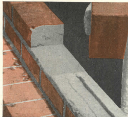
Then the excess mortar will fill the furrow and insure full bed joints.
