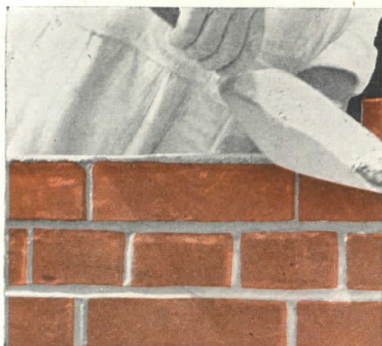
The mortar in this bed joint is spread too thin.
