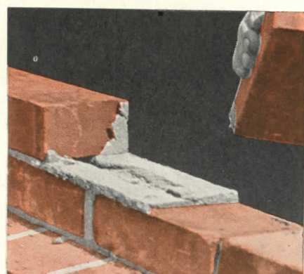
In either case there is not enough mortar in the bed joint to completely fill the furrow.
