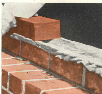
The furrow in this bed joint is too deep.
