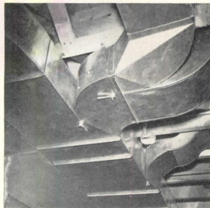
Aluminum ducts for heating or ventilating
