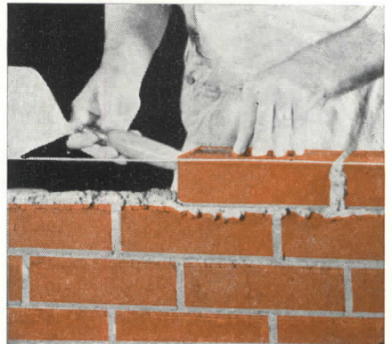
So the mortar dried out too much before the next course of brick was placed on top of it.
