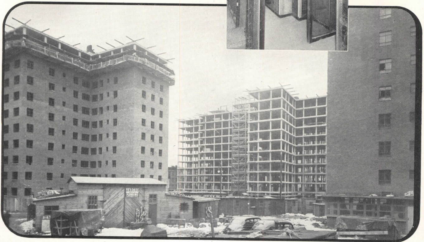
Truscon Diamond Metal Lath Used in Elliot Housing Project, New York City.
