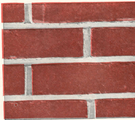
A struck joint leaves a shelf on which water collects.
