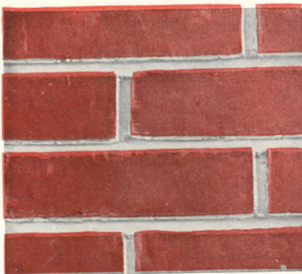
A weathered joint does not always pack the mortar against the top brick thoroughly.
