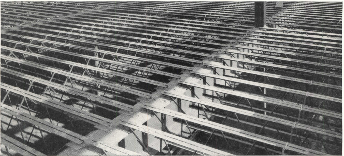
Architects: George and Henry W. Fox, Cleveland. Contractor: Sepper Construction Co., Cleveland. Joist Erector: Builders Structural Steel Co., Cleveland
