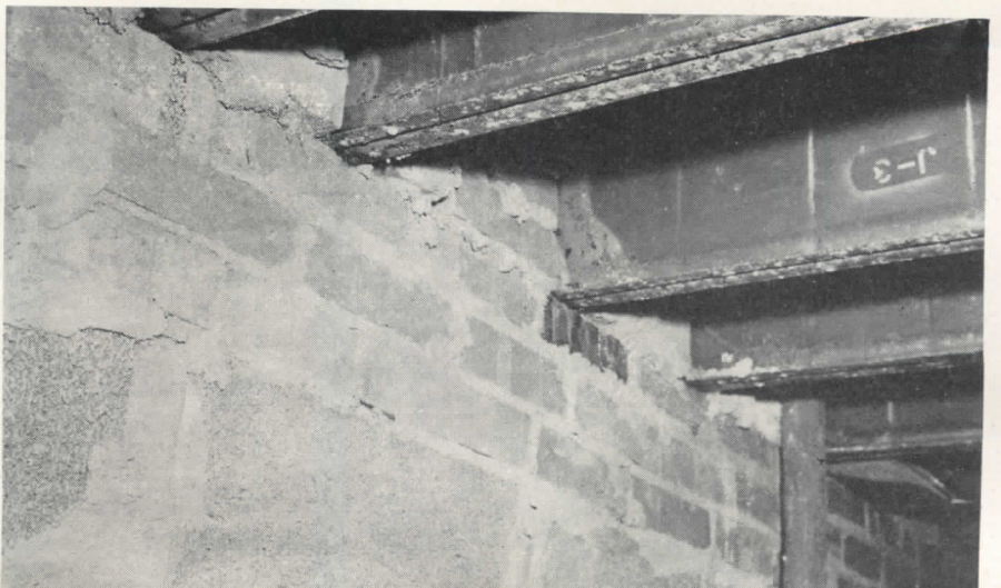
First-floor beams in apartment crawl spaces rusted at ends of webs and lower flanges
