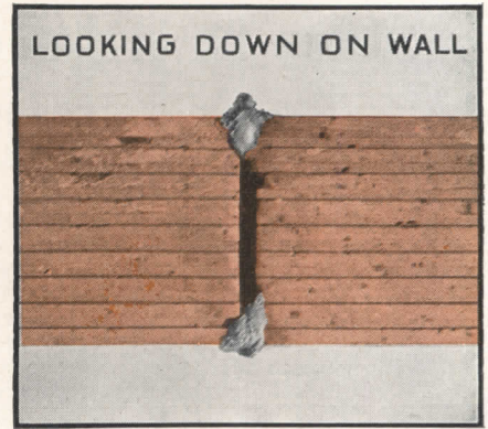
Enough mortar should be used to cause excess mortar to ooze out of the joints on both sides of the tile.
