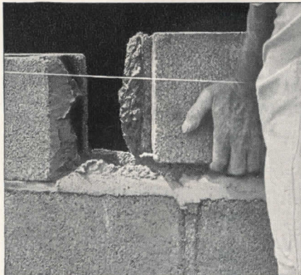
Method 2. A full head joint should be thrown onto one edge of the block already in place and also onto the opposite edge of the block to be placed.
