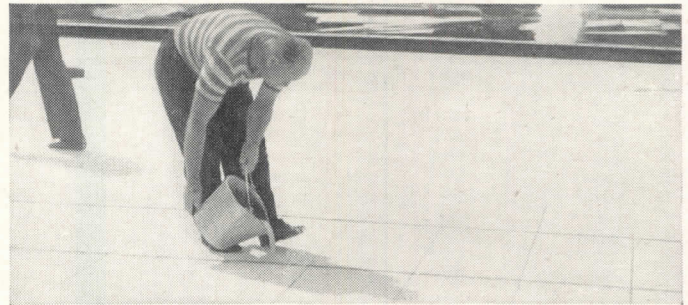
GROUTING is done when Kaylo Roof Tiles have been laid. After grouting is completed, roof is covered with conventional built-up asphalt or tar and gravel roofing. No additional insulation is necessary.
