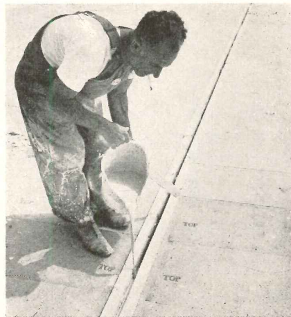
Left: lightweight, insulating roof tile is transported to work areas by wheelbarrow and then laid over structural steel members. Below: joints are grouted with mix of gauging plaster, vermiculite and water
