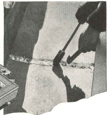
FOR PERMANENT PROTECTION, the old gutters have been replaced with gutters made of strong, corrosion-resistant and economical Monel Roofing Sheet. Here a worker solders a riveted seam in the gutter lining.
