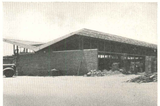
The four buildings comprising the modern design WESTSIDE UNION ELEMENTARY SCHOOL, Lancaster, California, utilize over 10,000 feet of Revere 1/2 inch type L hard temper Copper Water Tube in the radiant panel heating system. Architect: Frank Wynkoop; General Contractor: M. J. Brock & Sons; Heating Contractor: Ray Engineering Co.
