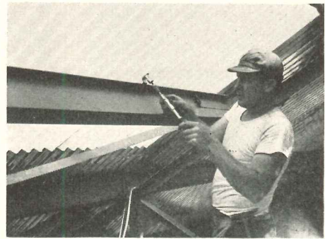
Left: skylights of white, translucent plastic, corrugated to match aluminum sheathing, admit daylight to University of Delaware field house. Above: close-up of plastic and center support
