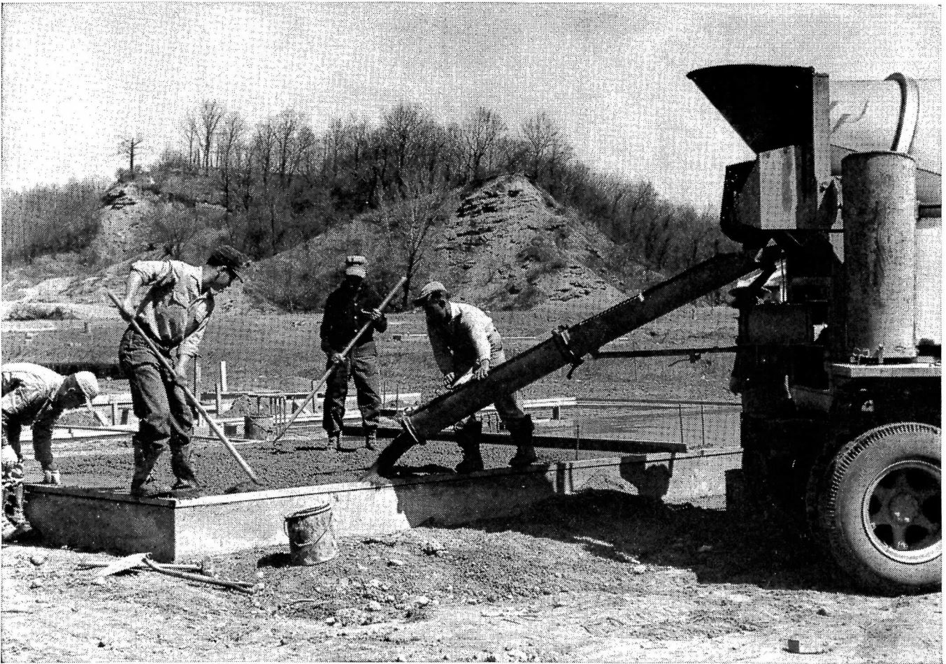
3. Next the slab is poured—and that's it! From experience National Homes finds it has protection from cold and damp for the lifetime of the house.
