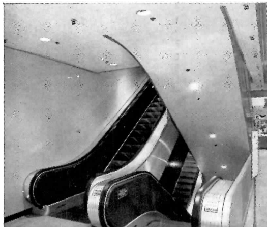
Supplementing Grinnell Ceiling Sprinklers at escalator stairwells is a special Grinnell Water Curtain System, which operates to keep smoke and hot gases from entering open floor areas.
