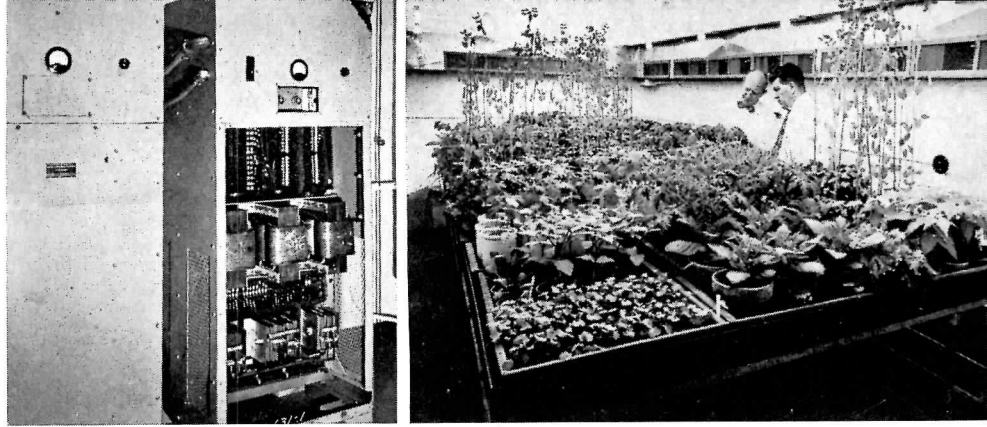
Installation at Dept. of Agriculture test station, Beltsville, Md. provides 2400 ft-candles 360 cycles. Frequency conversion supplied by magnetic multiplier, left
