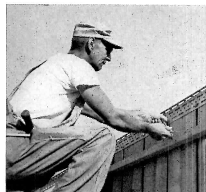
A single bolt at top and bottom of each panel secures them to horizontal steel angles attached to the sills
