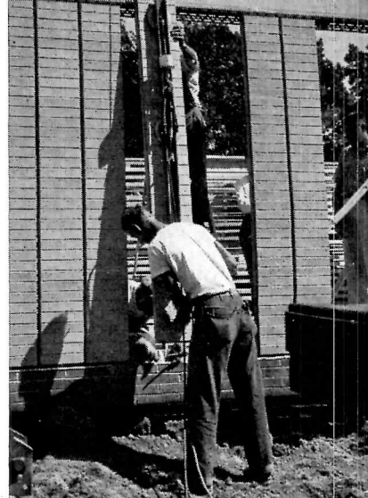
"SCR building panels," each made up of thirty-six norman-face brick set in stacked bond, are vacuum-lifted into place
