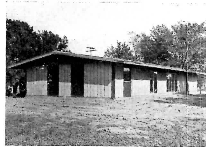
The brickwork completed — by five men in eight and a half hours, roof trusses are installed and finishing work begun
