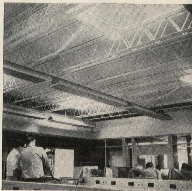
Truscon "O-T" Open Truss Steel Joists® are employed exclusively in North Hagerstown's new high school. Joists are covered by acoustical ceilings in all but a few laboratories—such as the electronics lab seen above—where possible increases or changes in electrical systems will require complete accessibility. Send coupon for "O-T" Steel Joist details.
