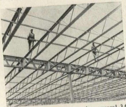
Workmen are shown carrying several 34' long lightweight box sections in the initial phase of the job. The sub-purlins are aligned in position with precision jigs and then fillet welded at each joist crossing.
