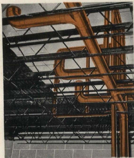
COPPER SANITARY DRAINAGE LINES roughed-in among structural members at Gower School. This space-saving installation would have been impracticable with heavy, bulky pipe requiring threaded or caulked joints.
