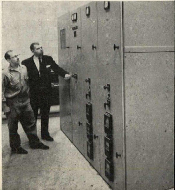
Walter Mack, The May Company Maintenance Supervisor, and E. E. Croushore, Jr., Westinghouse Construction Sales Engineer, take reading from ammeter on Westinghouse indoor metal-clad switchgear. Two 50 DH 150 air circuit breakers are used as feeders for the two Westinghouse 2000-kva power centers located at top of building. Utility company metering section is in far left compartment.
