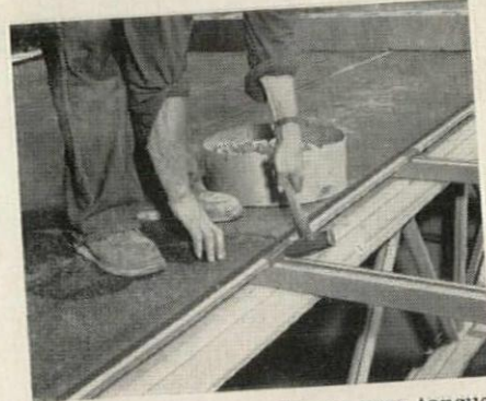
High speed clips are driven over tongue of plank. Tectum planks span three sub-purlins, giving added lateral strength. This operation is quickly accomplished.
