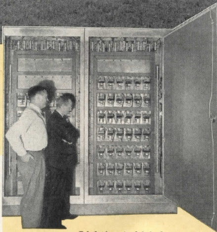
• Lighting (a high frequency system, 450 volts at 840 cps) in the Administration Building is controlled from this panel. Note space for future additions of Square D contactors as they're needed.
