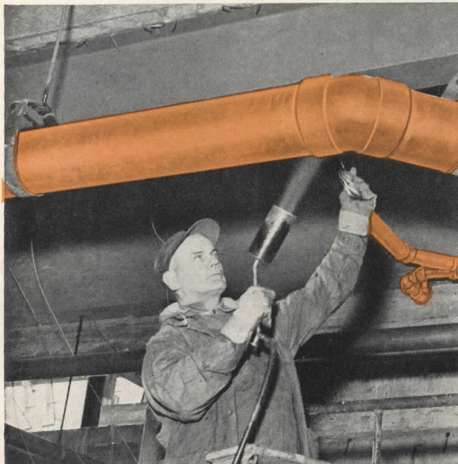
MAKING A SOLDER JOINT on an 8-inch copper soil and waste line — the largest size used in the drainage system. Solder-joint connections are one of the important reasons why copper tube systems are so much easier and faster to install.
