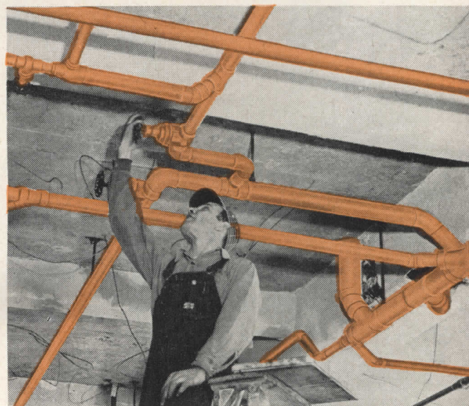
TESTING A VALVE on the hot-water supply system. Other copper tube lines in view are part of the sanitary drainage system, ranging in size from 1½ inches to 4 inches. Because connections are easily made, even in tight quarters, the lines can hug the ceiling.
