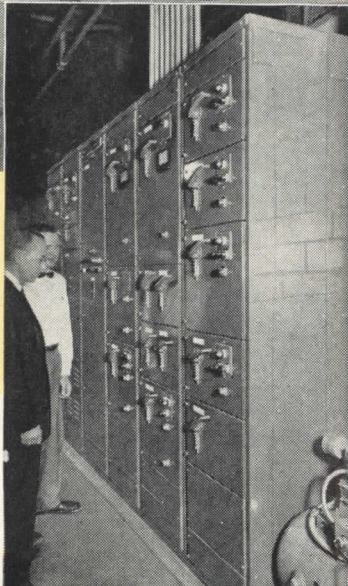
• This Square D control center in the Administration Building includes circuit breaker combination motor starters for the heat pump and air-handling equipment. Heat pump operation is automatically controlled through thermostats and programmed by clock system.
