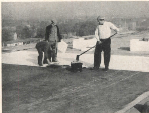
Figure 6. The roof is built up in the usual way after the polystyrene foam has been covered with a layer of asphalt-coated paper
