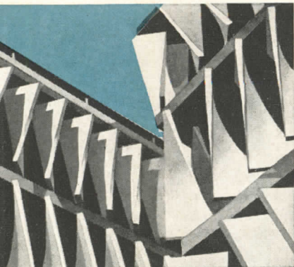
True hyperbolic paraboloids, 7'-4½" concrete panels have 90° twist, are 24" wide at top and base, 18" at waist.
