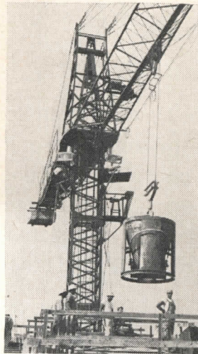
Crane is remote-controlled by one man from working deck with 3 1/2 lb. electronic panel. He is free to move to any part of the job, and to assist in loading and unloading.
