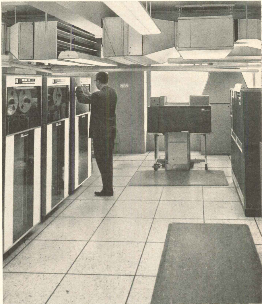
MELVILLE SHOE CORP., New York, N.Y. The computer room in this shoe company headquarters is air conditioned by a York "packaged" unit that maintains the temperature and humidity levels required for efficient computer operation. Contractor, Penguin Air Conditioning Corp., Brooklyn, N.Y.
