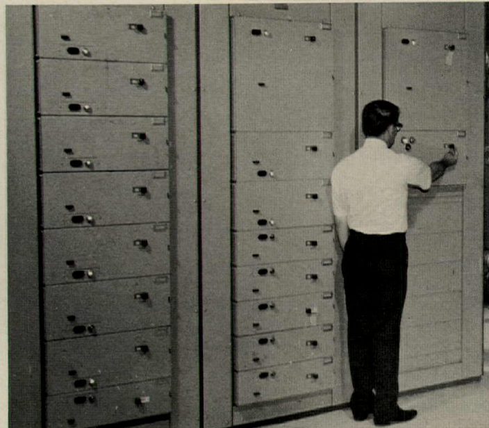
Main distribution panel, with pull-out type switches serving various sections of the 246-unit apartment project at Kenilworth.
