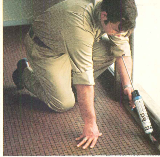
seal around tilework,
