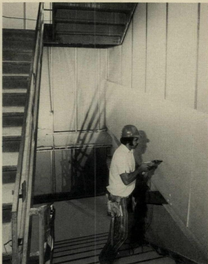
Alternate KW-621 System: For 2-hour stairwell enclosures, application is the same except that the second layer of ½" board is screwed to the studs from the stairwell side of the wall.
