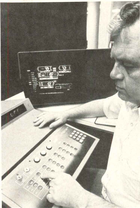
Console controls and monitors 65 buildings.
