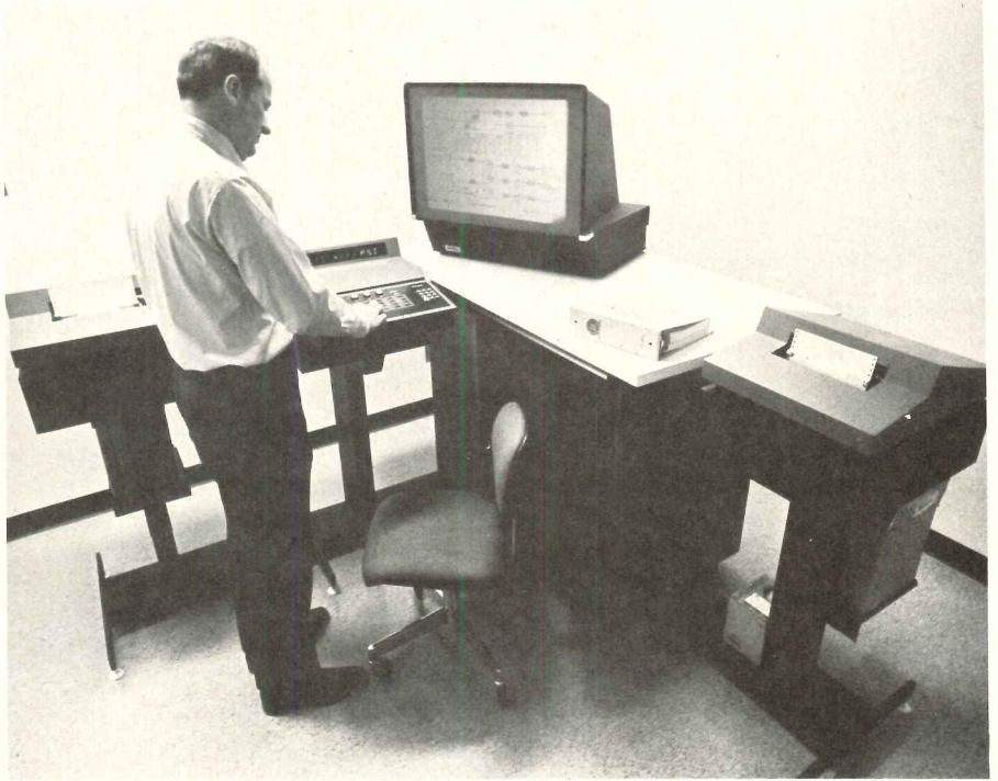
Automation control center in the Health Sciences building now handles a 10-building complex.
