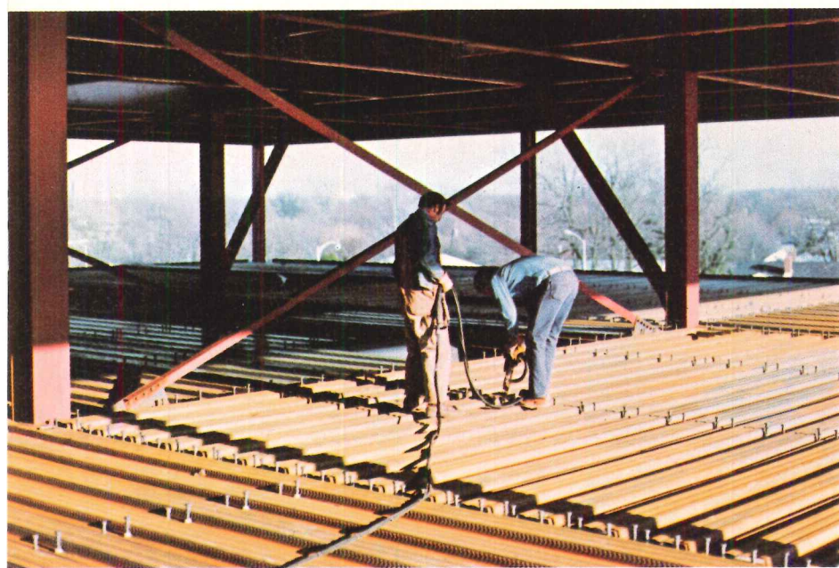
The floor system consists of a 3¼-in. lightweight composite concrete topping over 2-in. non-cellular composite steel deck. Floor-to-floor height is 12 ft. Bethlehem furnished all of the structural steel requirements for the building.
