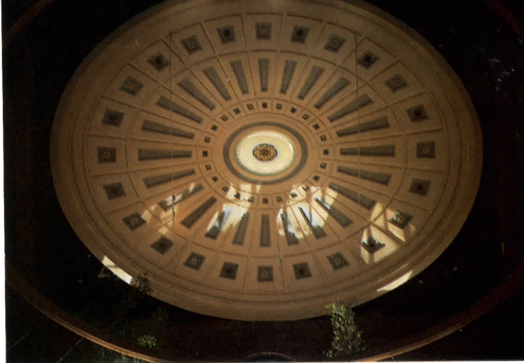
The great, elliptical, ribbed interior dome—long concealed by a hung ceiling—has been restored.
