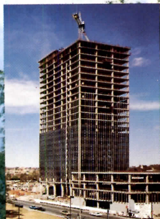
Ceco forming specialists formed a total of 834,000 square feet of flooring and averaged one completed 20,000 square foot floor every six working days.
