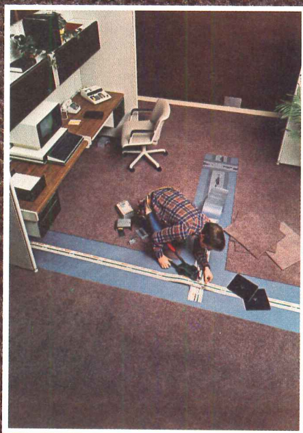
Flexway Undercarpet Systems for power, telephone and data transmission.
