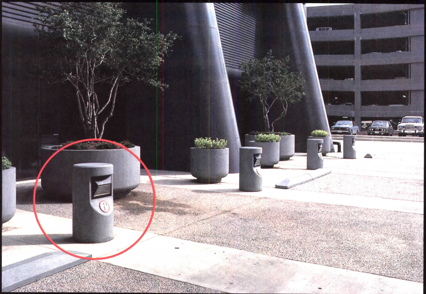
Kim Low Level Floodlights in precast concrete pedestals.
