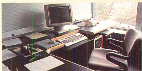
Installed at desktop level, the Wiremold perimeter raceway in this office handles both standard power and low voltage communications wiring.
