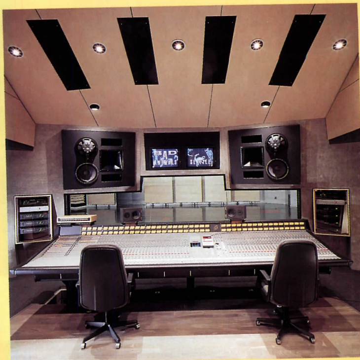
In the control room, acoustical absorption, reflection, and diffusion devices focus sound symmetrically.
