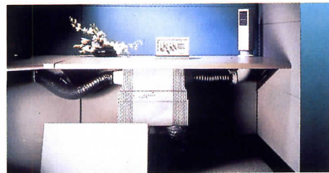
Johnson Controls' Personal Environment Module is the state of the art in task control but is bulky and needs base-building hvac.
