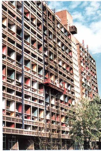
Work is being done on the facade of Le Corbusier's Maison Radieuse.
