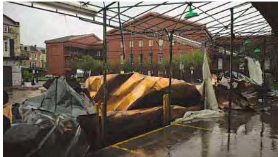
The copper roof was torn off New Orleans's 1835 Mint building (above). More damage reports are listed on page 48.
