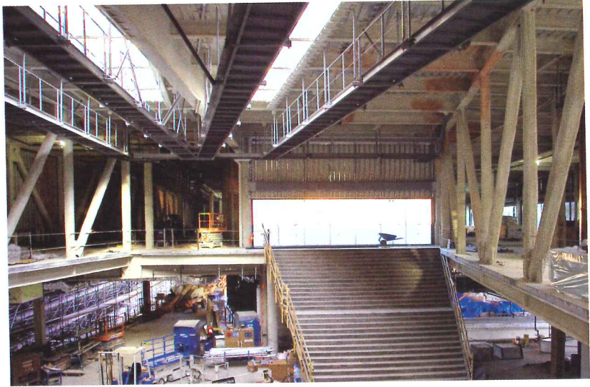
The owner’s desire for a museum with as many large, column-free spaces as possible resulted in long spans, one more than 90 feet, and trusses as deep as 20 feet.
