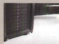
esd flooring systems
