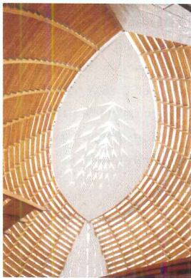
At the top of the cathedral, a steel compression ring holds the ribs around the perimeter of an oculus-shaped skylight (above). During construction, contractors supported the skylight on falsework (top) before beginning installation of the wood ribs.
