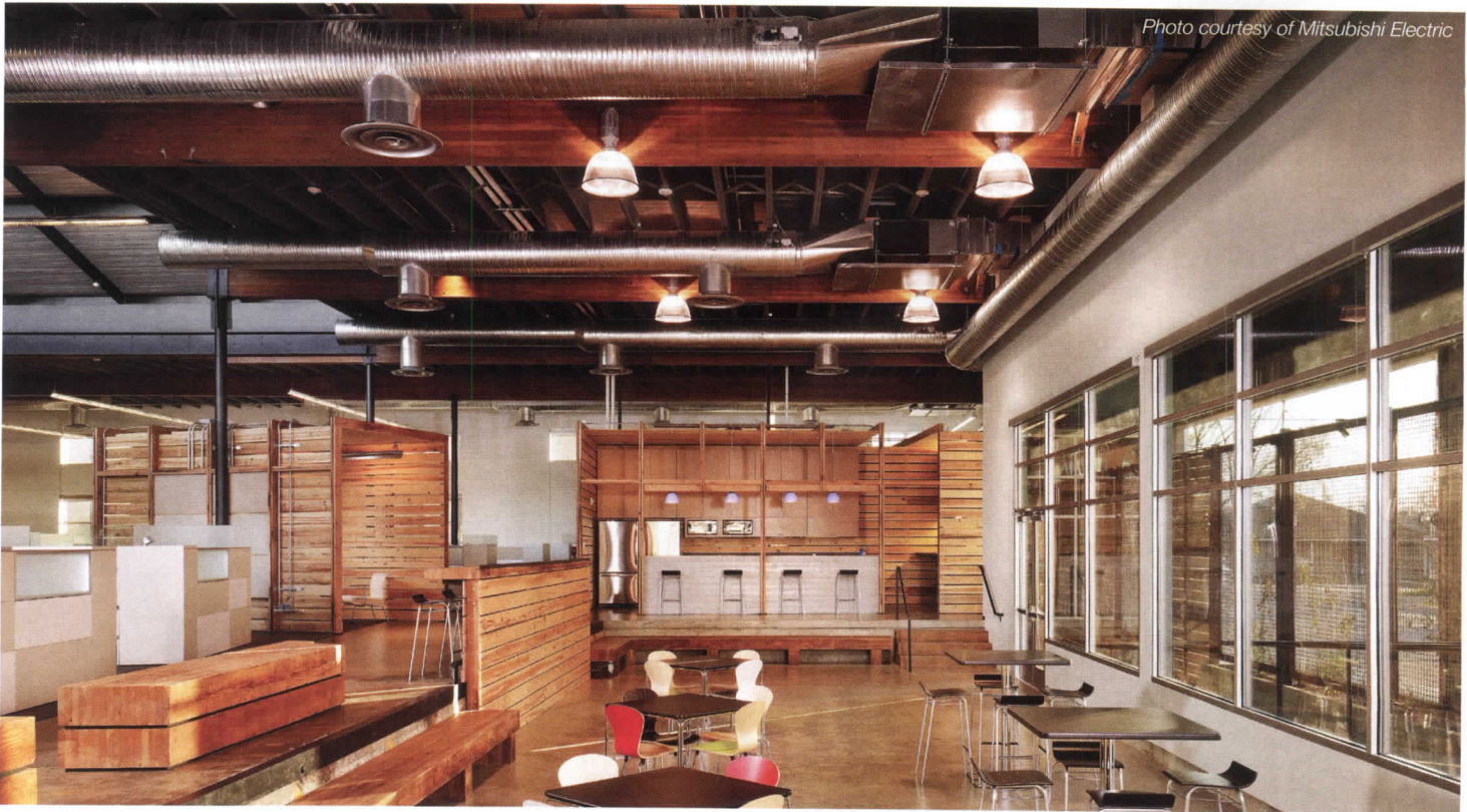
Exposed VRF system for a café demonstrates flexibility of placement and installation.
