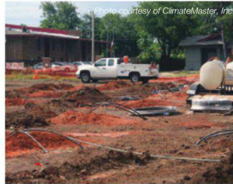
For the United Way’s headquarters for Central Oklahoma, a geothermal system was installed with 25 wells located beneath the new parking lot.
